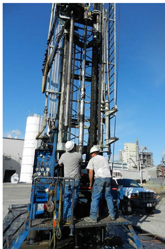
Technicians align a downhole packer and pressure /temperature monitoring system into the CO 2 injection well (Photo courtesy of Energy Solutions Inc. ).
